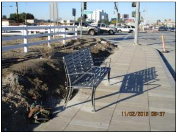
Bus Bench installed on Carson east of Figueroa
