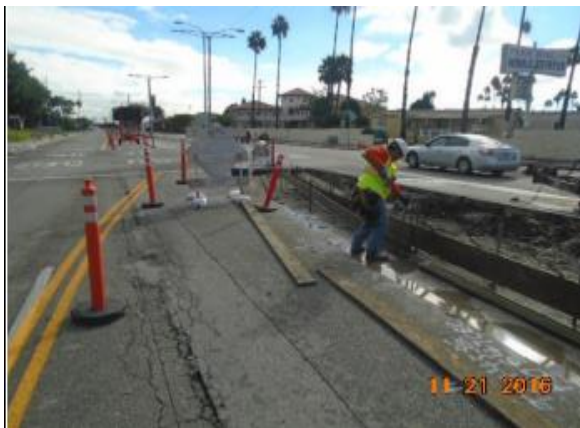
Powell forms curb and gutter for island at Carson St. and Civic Center
