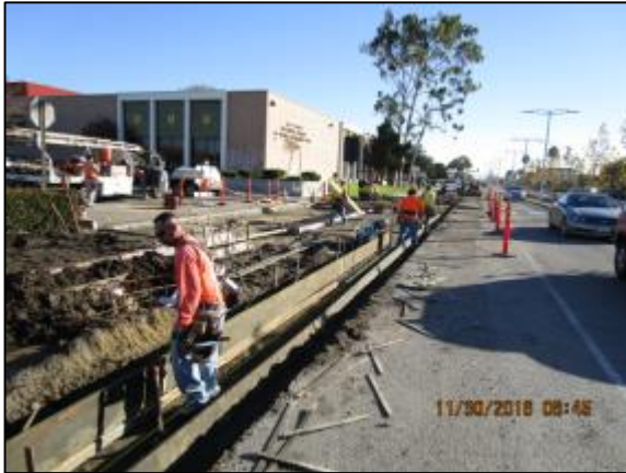
Forming curb and gutter on north side of Carson east of Main.
